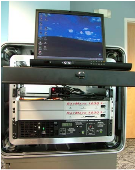
Figure 4a. Locus' ASF generation system. Starting from the bottom, a special power supply, two SatMate 1030s (one for each antenna type) and the PC with ASF software utility are installed in the rack. The GPS/WAAS receiver is mounted in the interior of the system.
