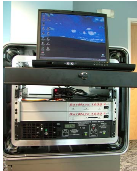
Figure 4a. Locus' ASF generation system. Starting from the bottom, a special power supply, two SatMate 1030s (one for each antenna type) and the PC with ASF software utility are installed in the rack. The GPS/WAAS receiver is mounted in the interior of the system.
